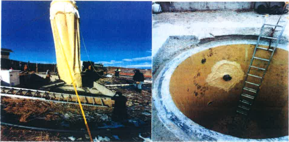
Cast in place liner bag being placed inside structure and after curing with steam and pressure.
