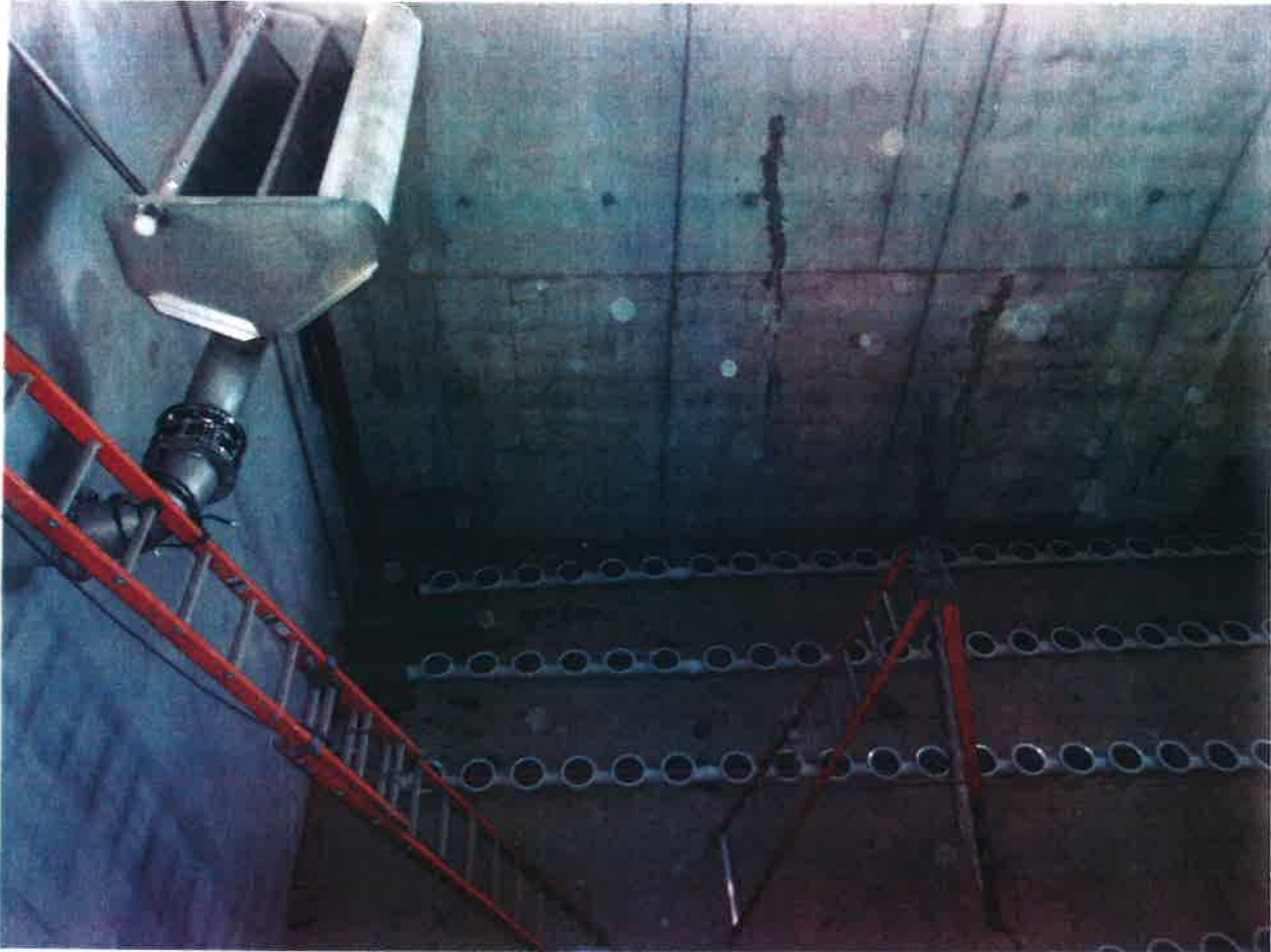
SBR Aeration and Decant assembly
