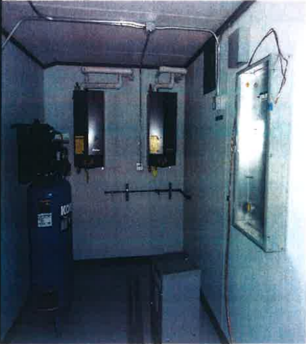
Mechanical and Control Room
